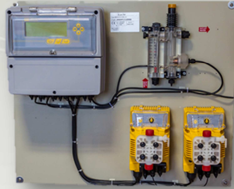
Helios 05 with 2 pumps
